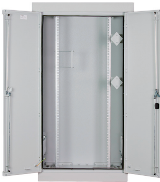
Street cabinets PU-7
